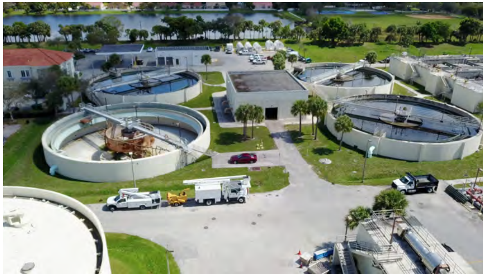
Wastewater Reclamation Facility
