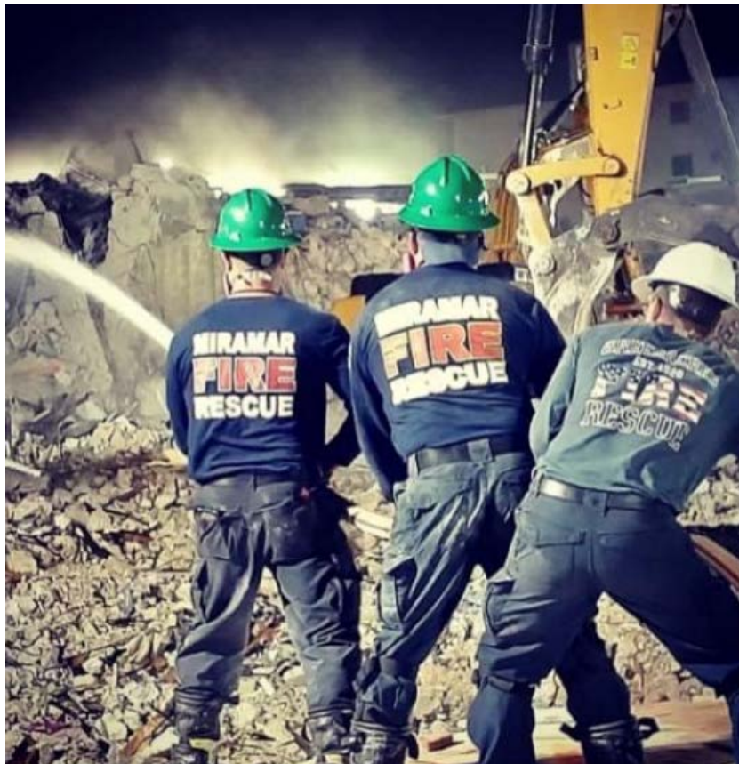
Assistance at Surfside (Miami-Dade County) Condominium Collapse
