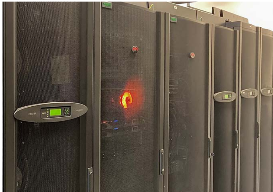
IT Server Racks
