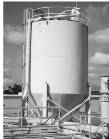
(b) Lime Silo at East WTP
